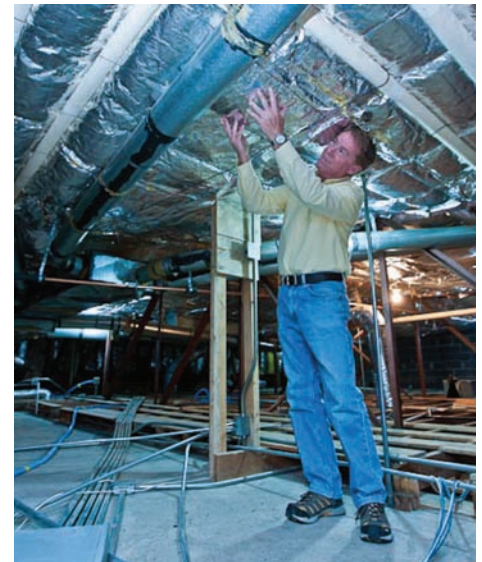
John Evans, Alpine Bank facilities officer, reviews work from a large insulation and air sealing project that improved the roof insulation factor from a leaky R-11 to a tight R-49. Photos by Todd Patrick
