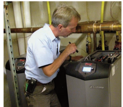
Left: Sunnyside Maintenance Manager Dean Crabb checks a setting on the two new 93 percent efficient boilers in the main building. Photos by Suzie Romig
