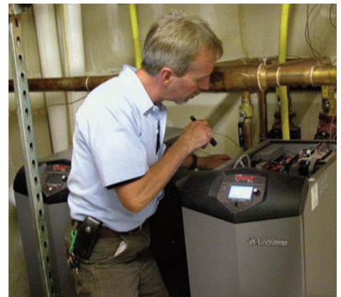
Left: Sunnyside Maintenance Manager Dean Crabb checks a setting on the two new 93 percent efficient boilers in the main building. Photos by Suzie Romig
